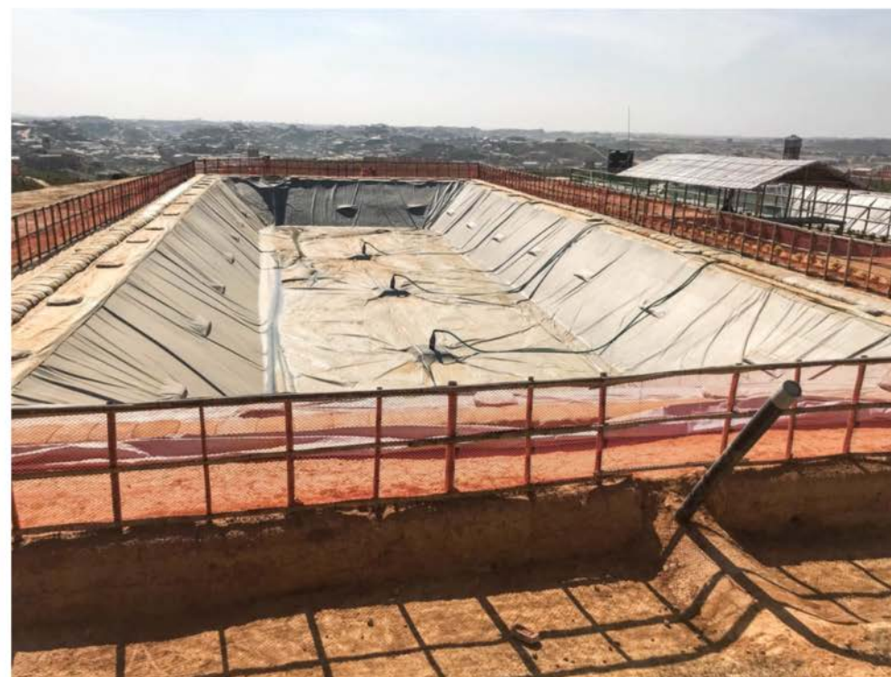
The human waste treatment facility under construction at the refugee settlement near Kutupalong, Bangladesh. © UNHCR/Firas Al-Khateeb
