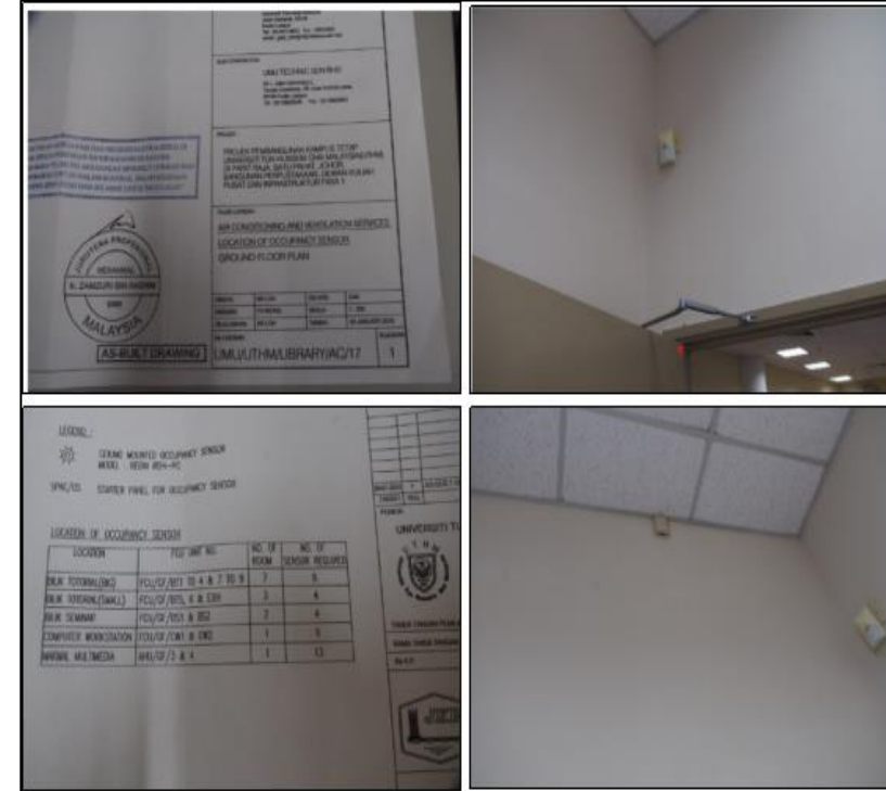
The automatic lighting sensors were installed at the Tunku Tun Aminah Library (L2 element)
