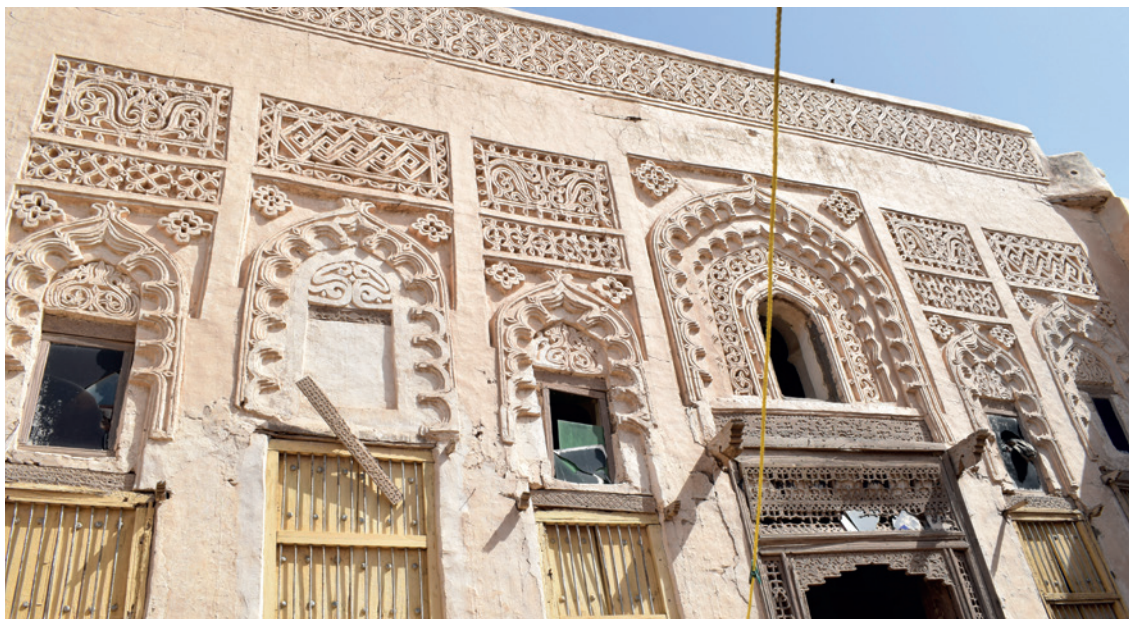
▲ FAÇADE OF HAWAIJI HOUSE, PART OF THE WORLD HERITAGE PROPERTY OF THE 'HISTORIC TOWN OF ZABID' (YEMEN), DAMAGED BY THE TORRENTIAL RAIN AND FLOODING IN AUGUST 2019 © UNESCO
