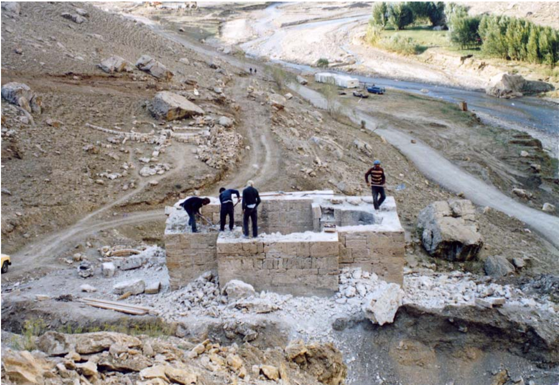
The Dzordzor Chapel in its original emplacement. The dismantling of the monument. View towards the SSW.
