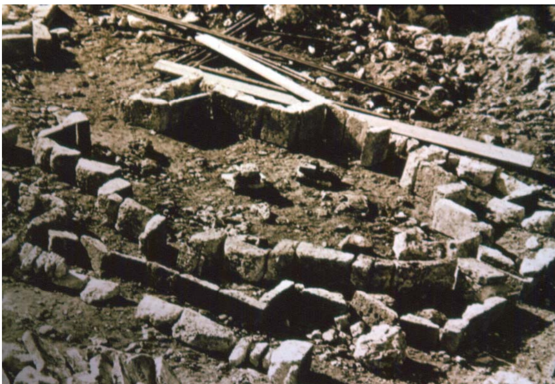
The Dzordzor Chapel. A dismantled layer of the monument laid on the ground for numeration and transportation to the new emplacement.
