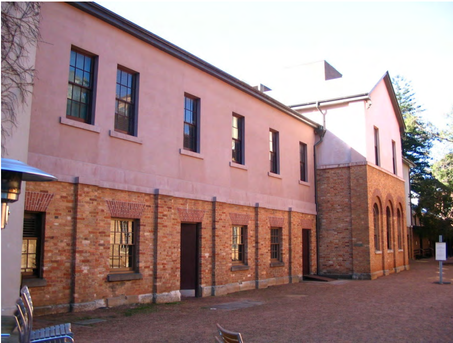
Figure 16: Current condition of the site – detail of façade of brick northern range of buildings showing state of conservation of exposed brick facades with stone footings (ground level) and rendered brick (upper level), window treatments and graveled surface of courtyard, all in good to very good condition.
