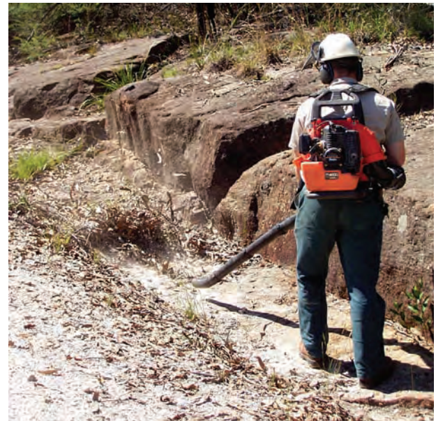
Ongoing maintenance works to remove vegetation growth at Old Great North Road.
