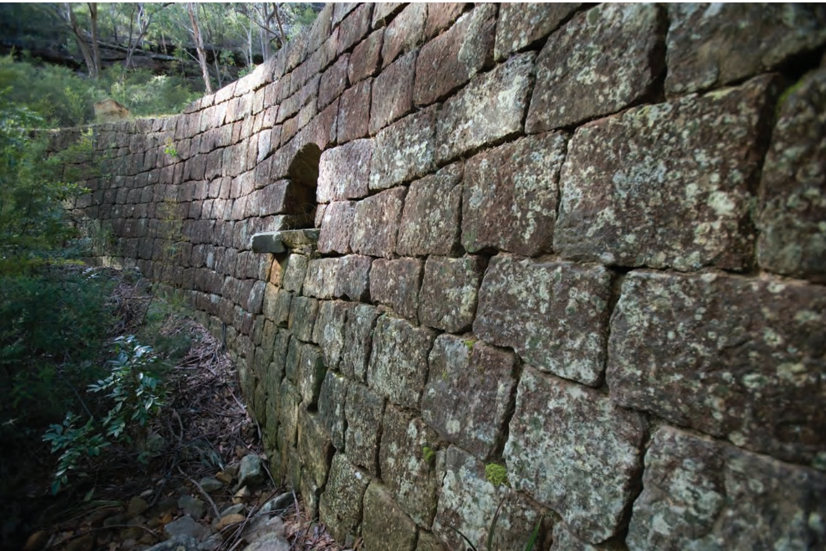
Convicts quarried thousands of sandstone blocks from cliffs to form massive retaining walls.
