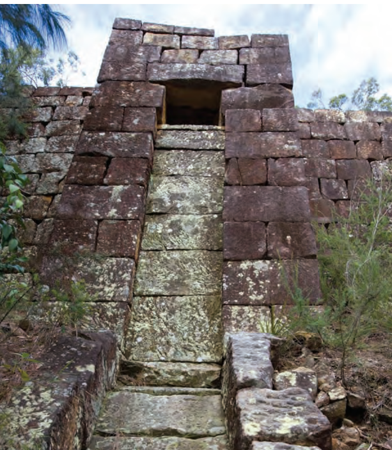
Old Great North Road is a rare intact example of early colonial road engineering undertaken by convict labour.
