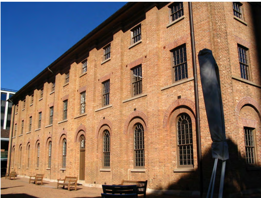
Figure 17: Current condition of the site – detail of façade of and north-facing wall of brick central Barracks building showing state of conservation of exposed brick facades with stone footings (ground level), window treatments and graveled surface of courtyard, all in good to very good condition.
