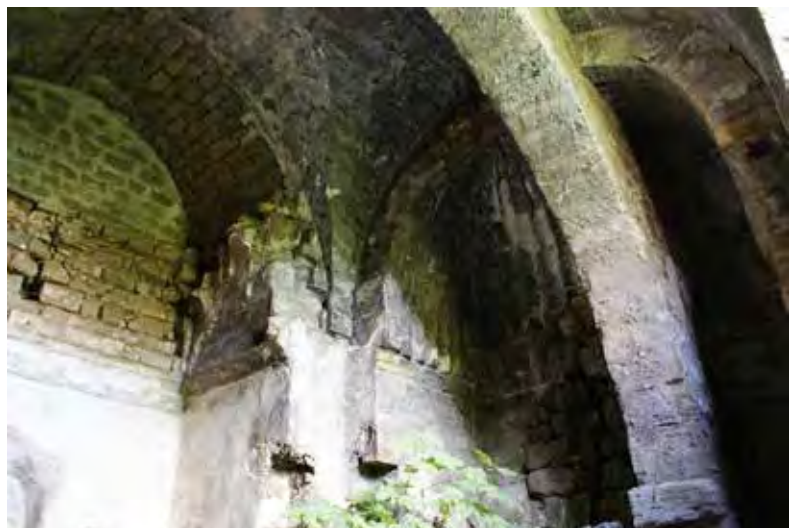
Palermo, Scibene, interior of the room with iwàn, XII century, second half
