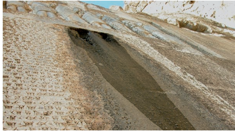
Algae and lichen around seepage water.
