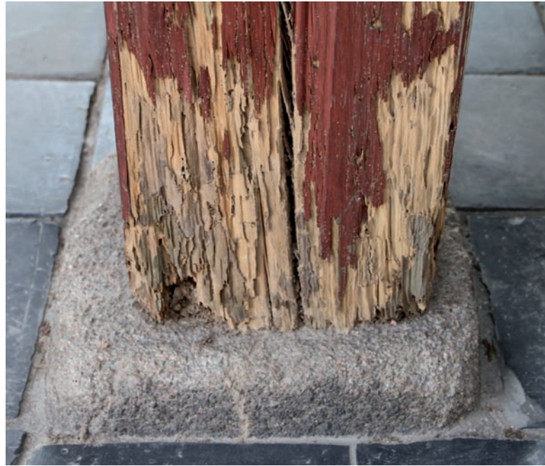
Damage on wooden structures caused by termites.
